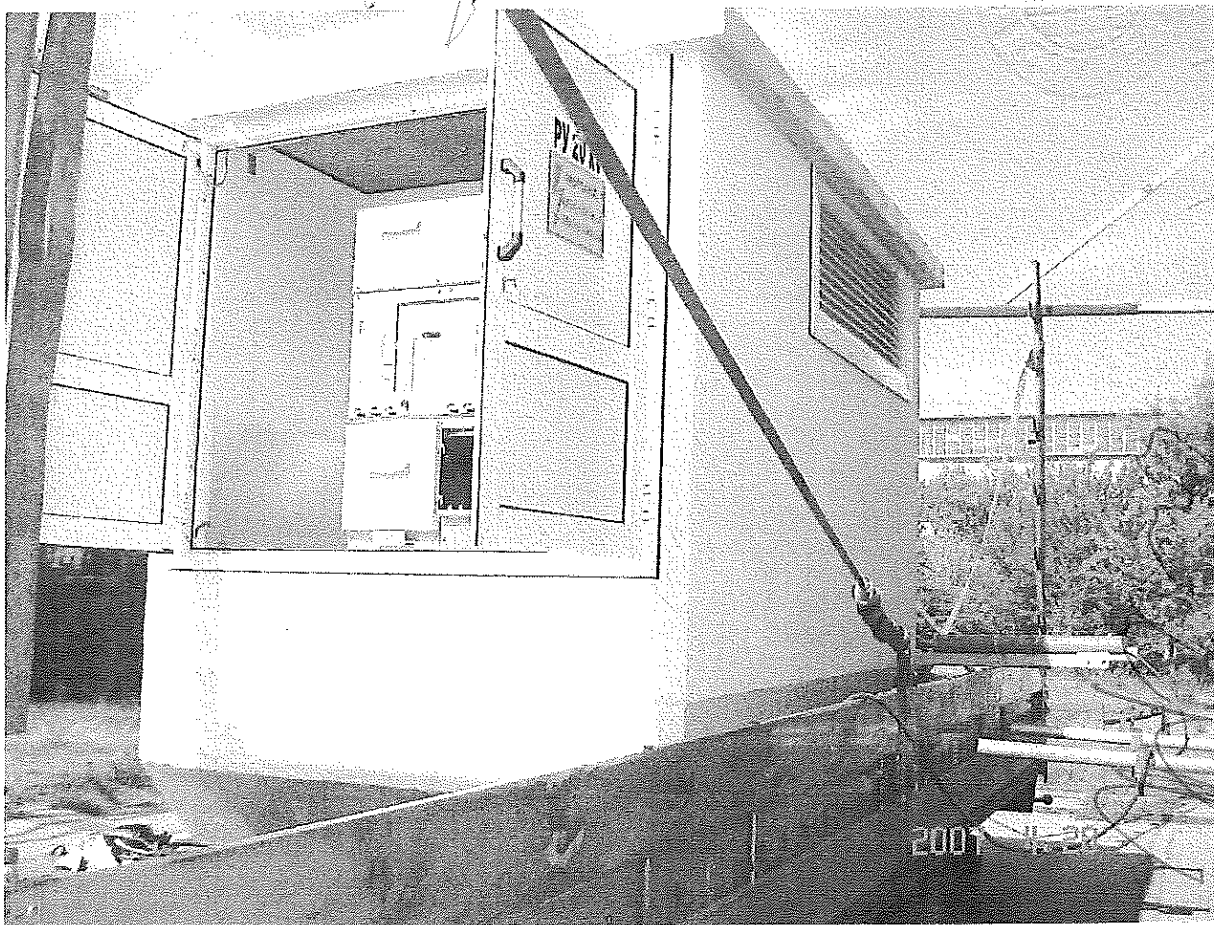
Photo 1 – Aspect of the complete transformer substation in the test circuit
